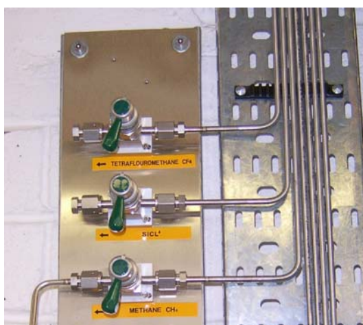
Figure 11 Gas supply point-of-use valves
